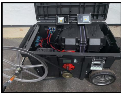
Figure 15: Front view of generator with open lid, featuring lights
